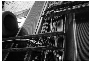
Rusting of metallic trays in a corrosive environment
